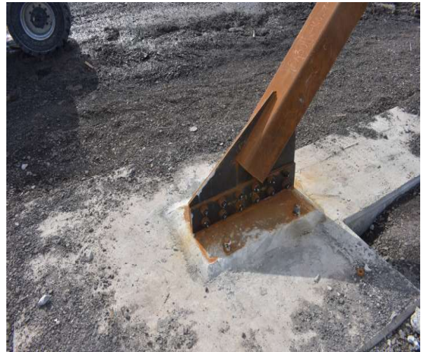
Steel frame gantry for traffic
